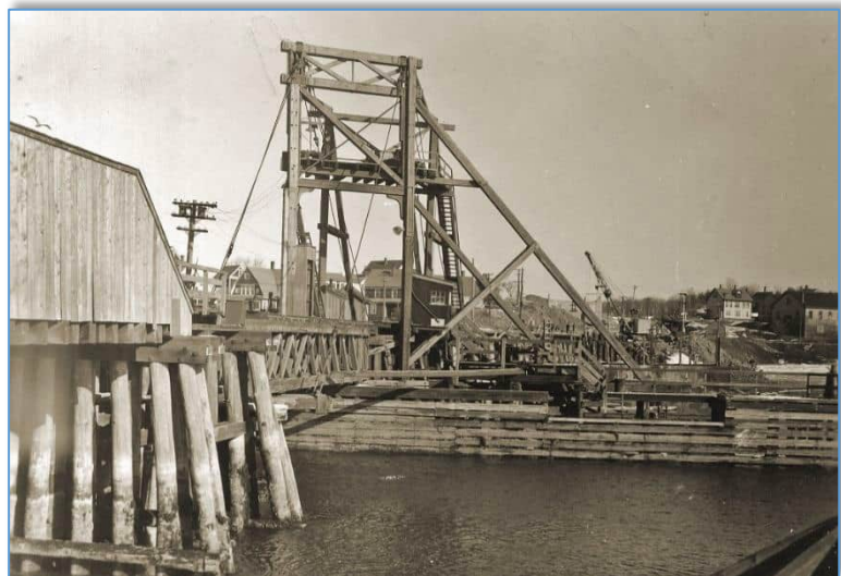
Photo of the main draw span near the Kittery shore taken in 1939 during construction of the Interstate Bridge that was being built to replace it. At center is the timber-framed shear leg (or shear pole) lifting tower from which the swing span was suspended when open. A single set of shear legs are supported with wire rope guys attached to the top of the tower and back to anchor points on the bridge. Here a second set of shear legs is used forming a square tower carrying an elevated platform on which the hoisting machinery is mounted (see additional photos below). Pile bents extend out perpendicular to the bridge on the east side of the draw opening, as a fender system and to support the diagonal shear leg that assists in carrying the load of the open draw span. The draw span consisting of a timber deck truss, visible left of center supported by lift cables, is anchored to a pivot at the end under the shear tower and swings out at a right angle over the adjacent fender system. The draw above was installed in 1913 and took ten to twelve men 30 minutes or more to open and close, often causing train delays and long traffic backups. The problem grew worse each year and in 1918 the B&M finally installed electric motors to operate the draw, something they had done on their Dover Point Bridge and Portland draws in 1909. Courtesy of Portsmouth Athenaeum.
