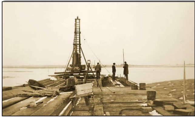
Cowles & Childs Construction Co. driving piles for the bridge in 1901. The 4,923-foot structure stood on 5,270 oak piles. It was completed in one year by three steam pile drivers. A 30-foot bascule draw spanned the river channel near the middle of the bridge. Photo courtesy of Lane Memorial Library.
