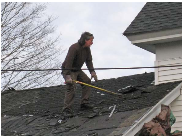
Building improvements at the museum continue with a new roof installation on the 1960s wing and Tuck Hall.
