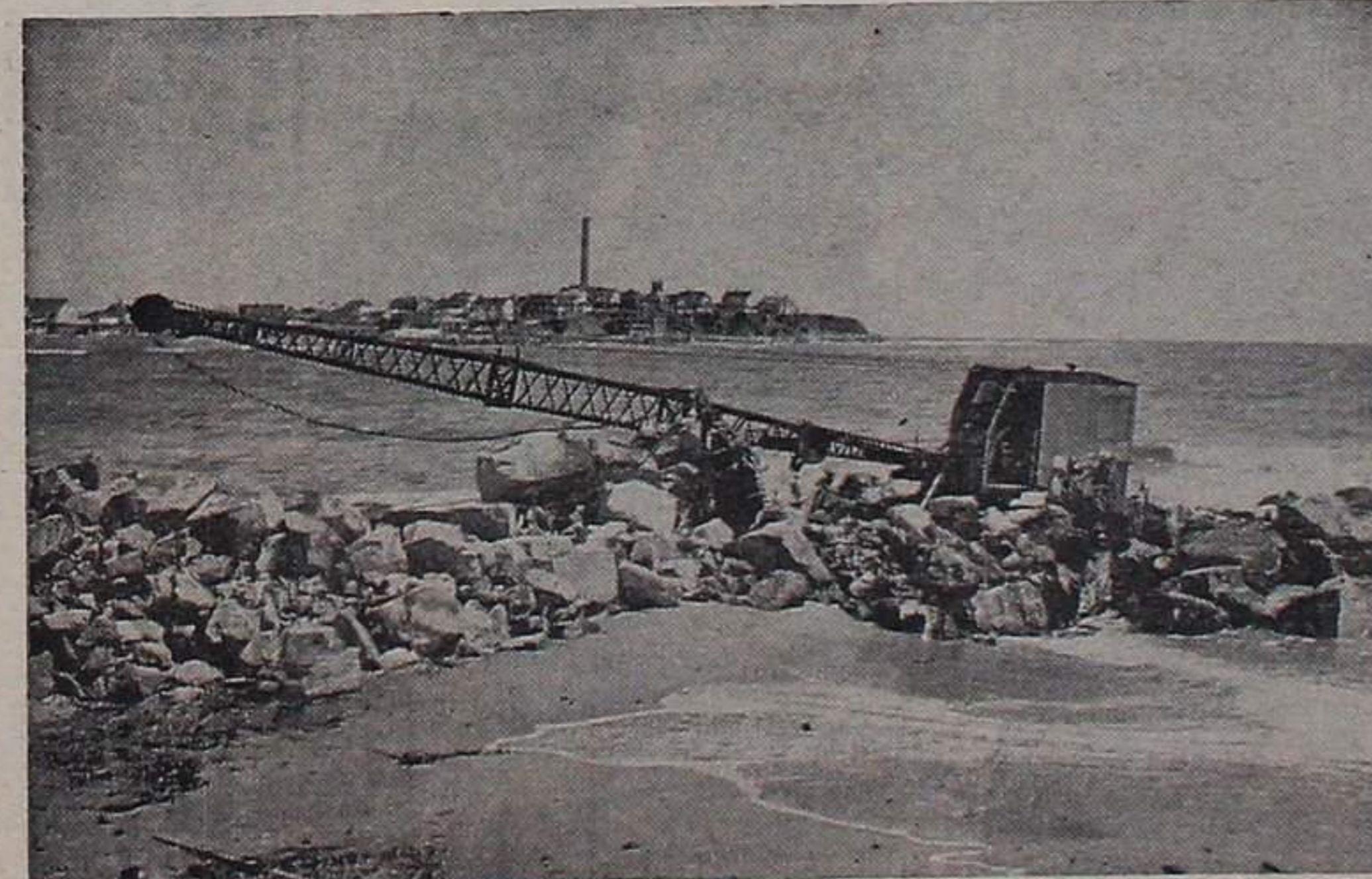
ONE PHASE OF THE HARBOR IMPROVEMENT construction for Hampton Beach and River has been completed with the erection of a stone groin off Church Street, shown above several months ago in the first stages of construction. Purpose of the groin is to prevent sand from washing off the north end of the Beach. Randall Photo
