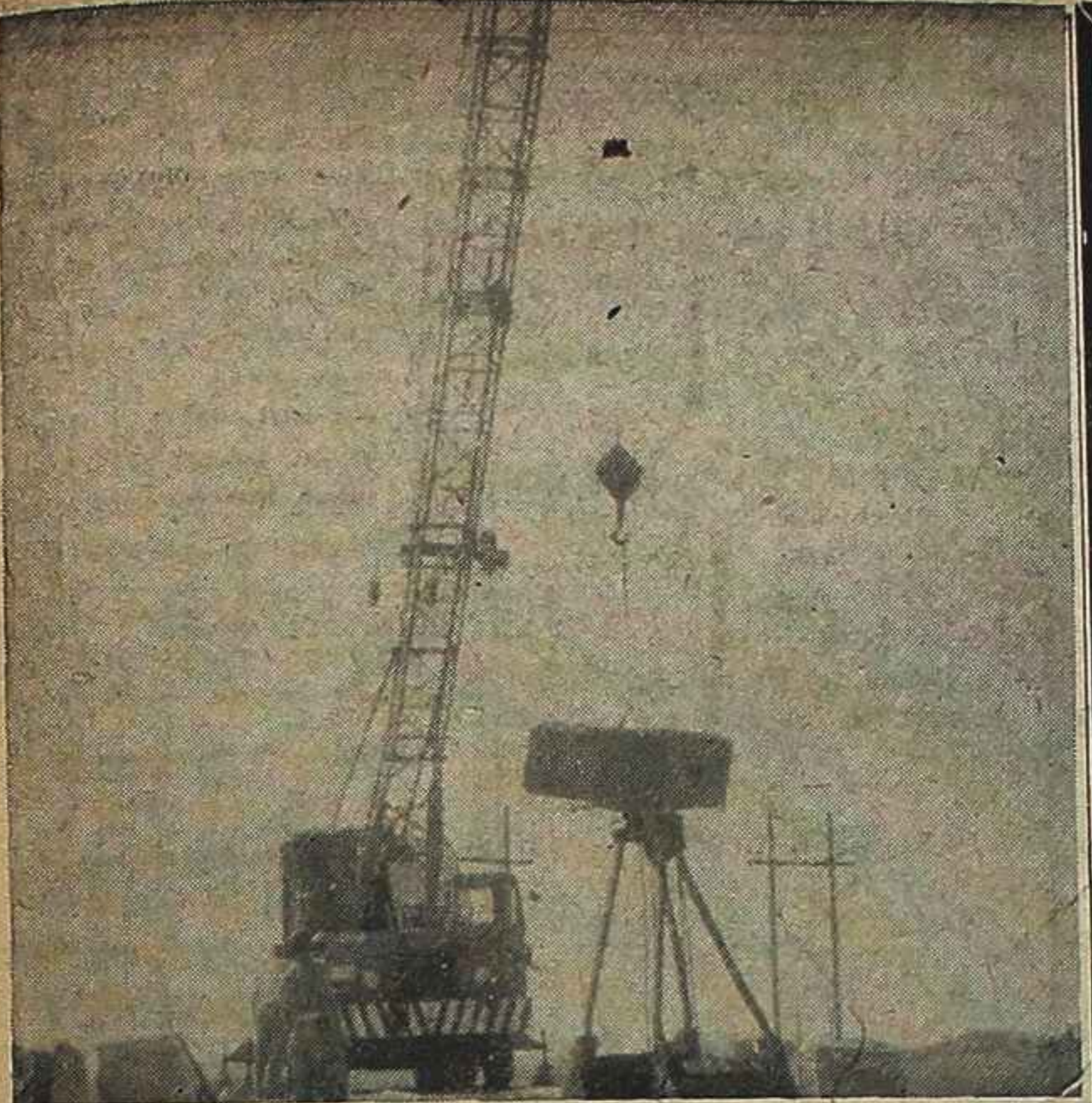
TIDE MILL BRIDGE construction should be completed in about two months it was reported this week as State Highway crews (above) began driving pilings for the $21,000 span which will provide a new link between the town and beach.
