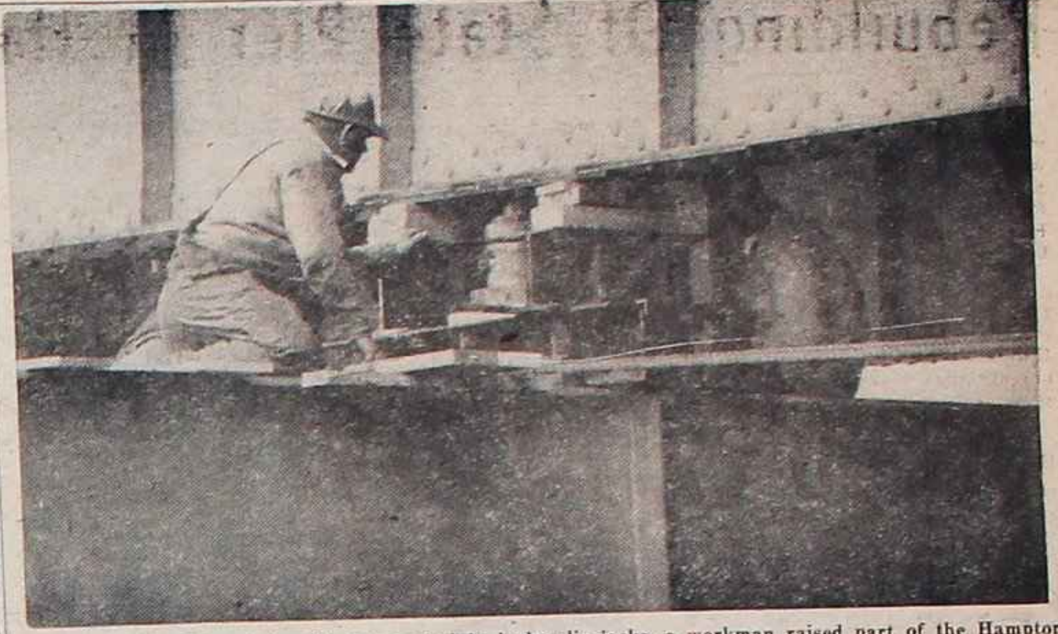
WITH ONE HAND and the aid of one of eight hydraulic jacks, a workman raised part of the Hampton River toll bridge back to its original position Friday, June 7. Following the completion of the jacking of the span which dropped 5 inches on May 4th, the bridge was reopened to traffic not exceeding three gross tons.
