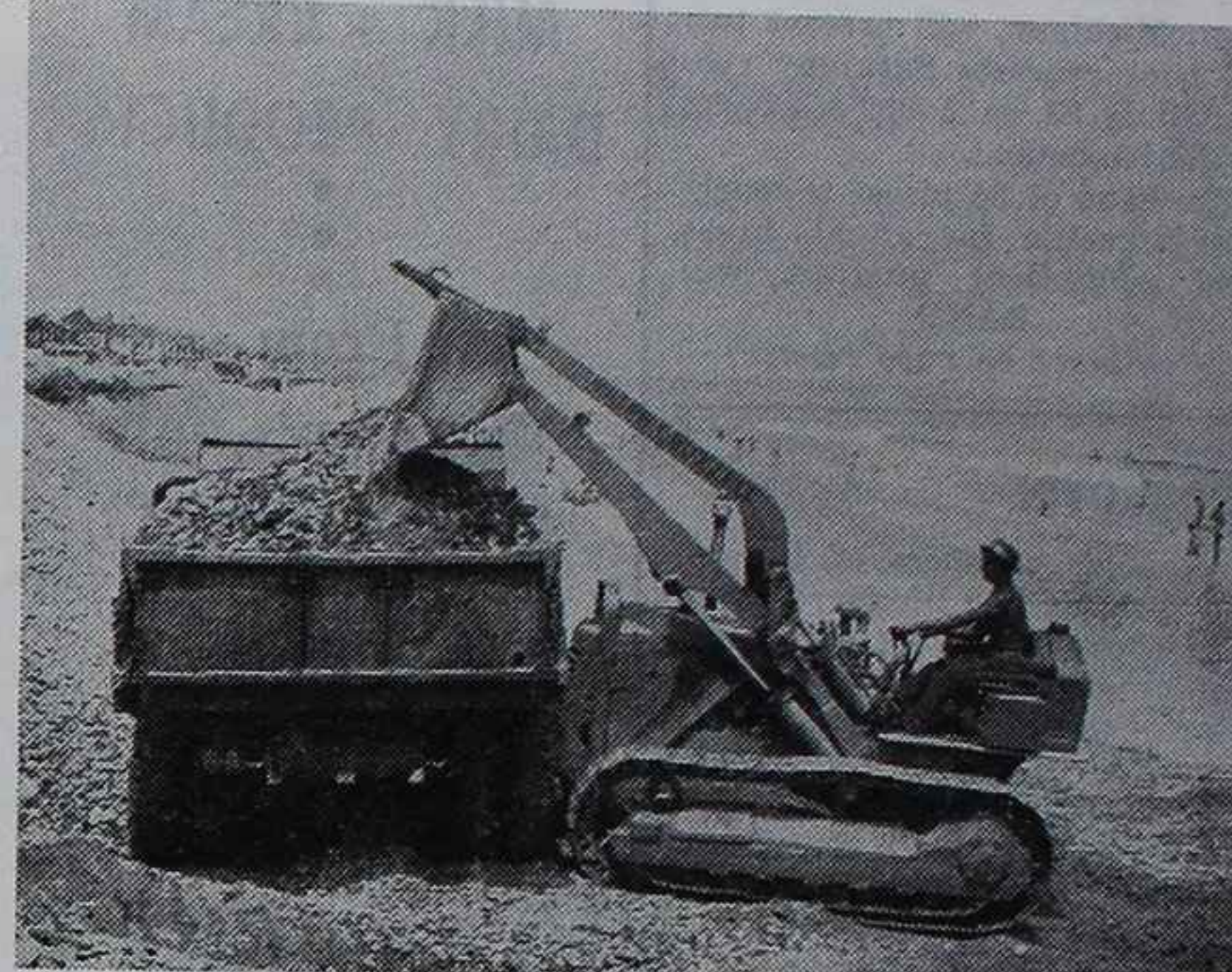
BORROWING STONE FILL from the protective banking north of Great Boar's Head, at the head of 5th street, a scoop shovel is pictured above loading a truck. The material is hauled to fill the cavity between the finished concrete seawall and the highway south of the Head. Seawall construction in the above-pictured section is expected to start early next month.
